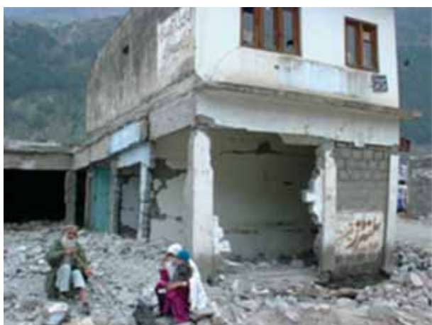
Fig. 5: Earthquake damage, 2006 Barakot, Pakistan
