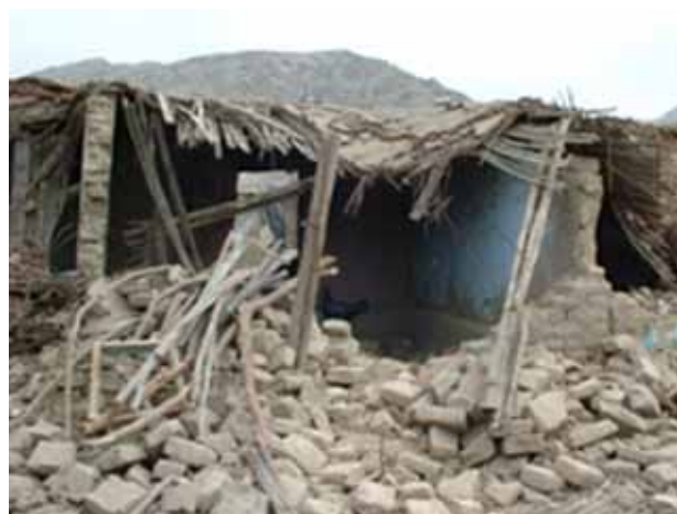
Fig. 10: Damage of rural house, 2007 by UN (suburb, Ica)
