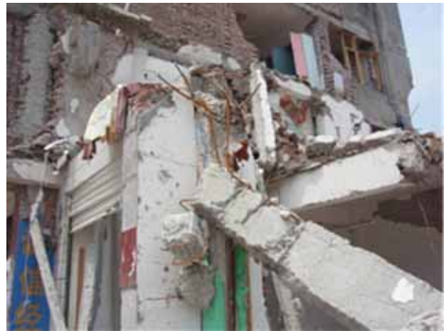
Fig. 13: Damage of RC structure, 2008 by UN (Sichuan)
