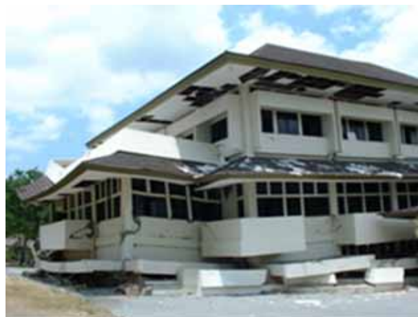
Fig. 6: Earthquake damage, 2006 Bantul, Indonesia
