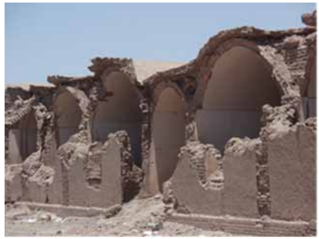
Fig. 20: Damage of adobe structure, 2003 (Bam, Iran)
