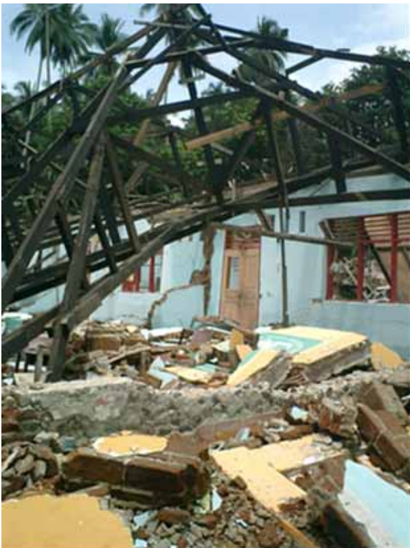
Fig. 15: Damage of non-engineered school, 2009 (Padang)
