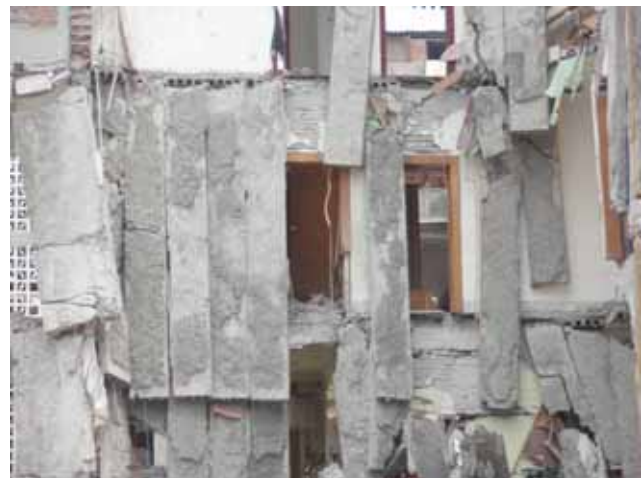
Fig. 22: Damage by Wenchuan Earthquake, 2008 (China)
