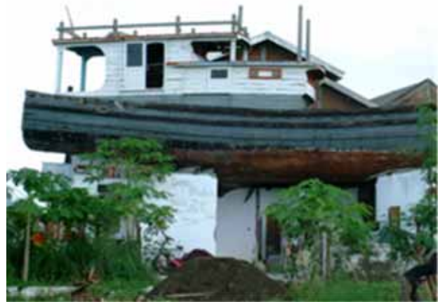
Fig. 3 Remaining Ship on the Roof, 2007 Aceh, Indonesia
