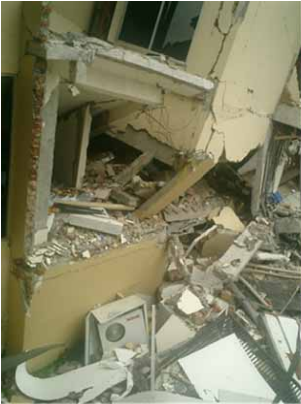
Fig. 14: Damage of RC building, 2009 (Padang, Indonesia)
