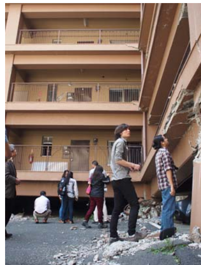
Damaged building in Kumamoto
