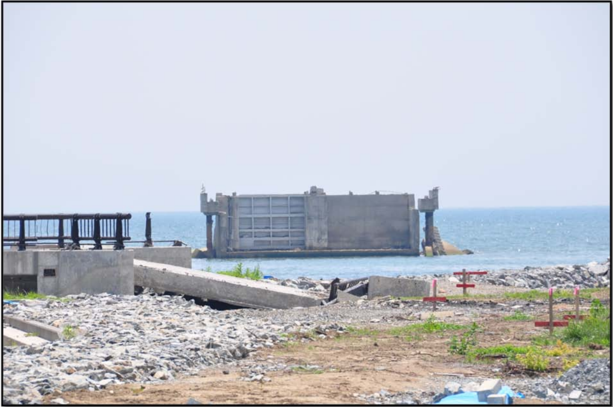
Figure 11: Damaged flood gate caused by tsunami at Rikuzen-Takata. (Photo taken by Fatimah Zaharah )
