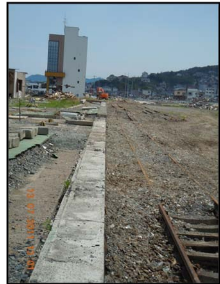
Figure 13: Damaged railway. This is very important transport in Ofunato city. (Photo taken by Mazni Azis)
