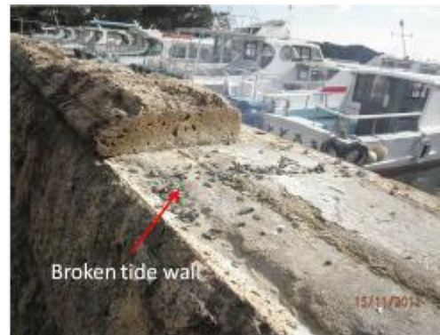
Figure 2.2. Broken tide wall in Matsushima.
