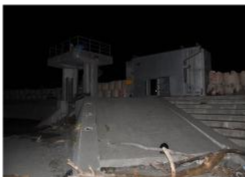
Figure 3.4. The broken sea wall at Shirahama Beach.
