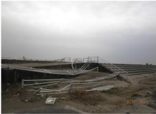
Figure 1.2. The broken sea wall in Arahama Beach.
