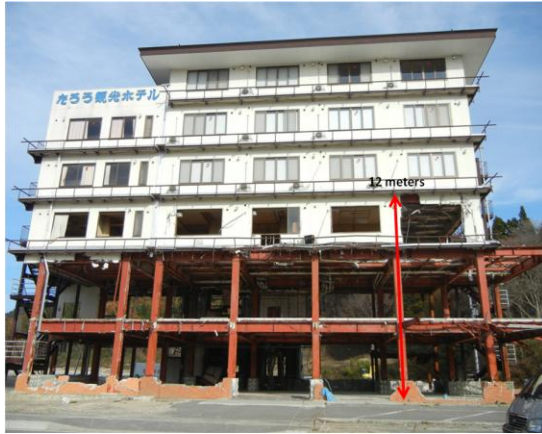
Figure 5.3. The damaged building in Taro.
