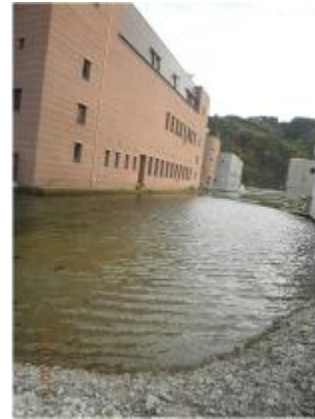
Figure 2.6. Sea water covering the road around the building describes the land subsidence.
