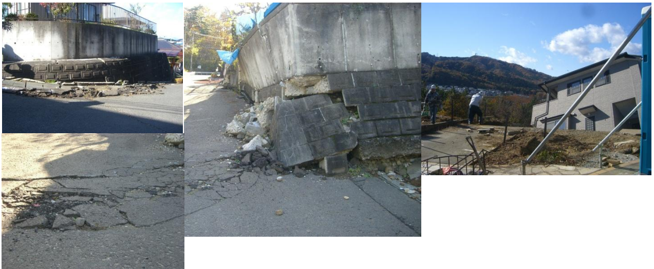
Figure 9. Damage of Retaining Wall, House Movement and Tilting by Sliding and Ground Transformation
