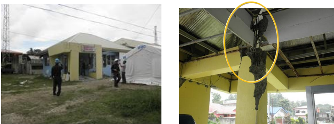
Figure 12. An example of improper structural design (by the earthquake) (Left) Exterior view of District Health Care Center of Sagbayan, (Right) connection of a column and beams
