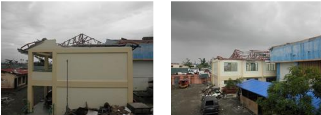
Figure 14 Tanauan National High School in Leyte (by the typhoon): (Left) Collapsed gable walls of CHB. (Right) Roof truss heavily damaged without sufficient reinforcement in longitudinal direction
