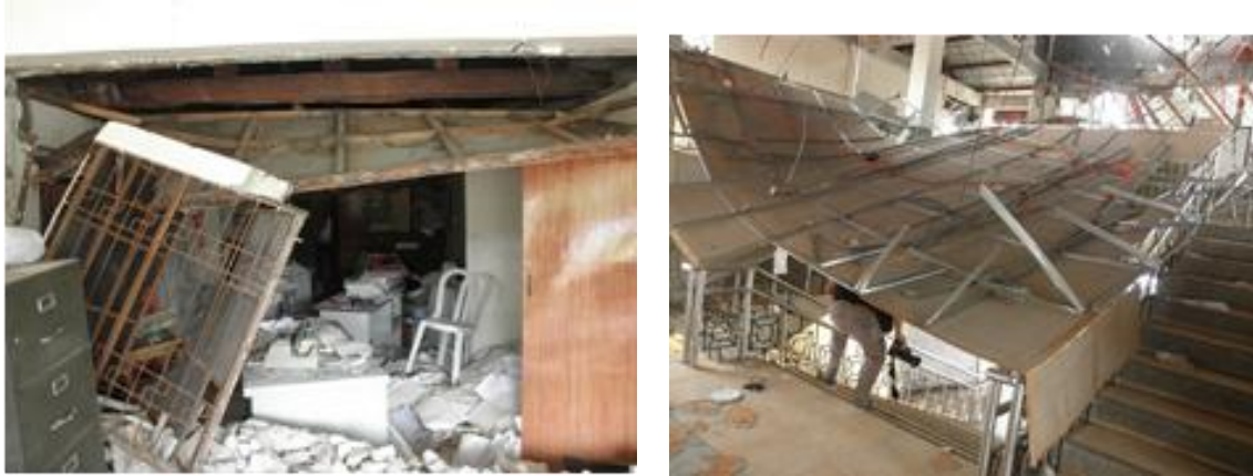
Figure 23 Examples of improper fixing of ceiling boards (by the earthquake): (Left) Sagbayan Municipal Building, (Right) Market Building in Loon.
