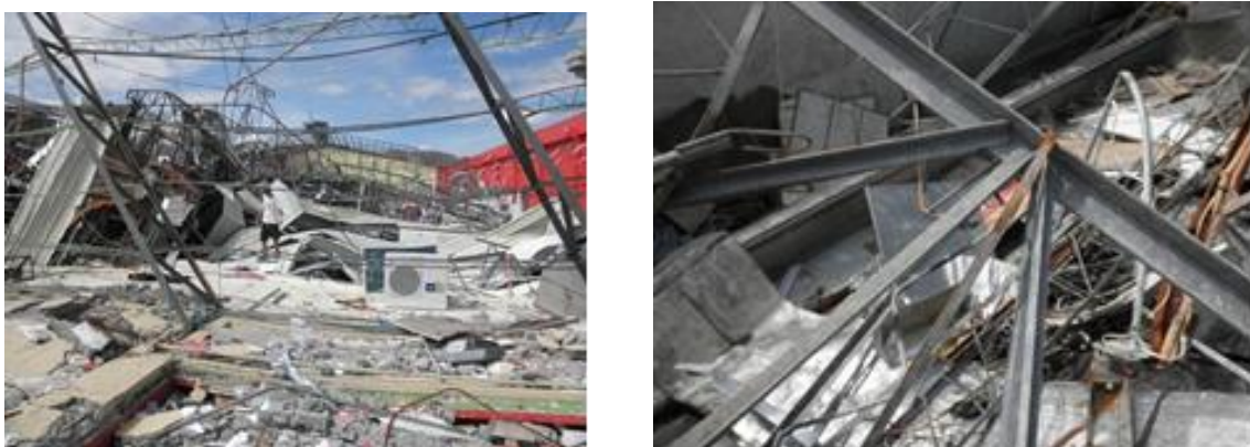
Figure 15 Supermarket Metro in Leyte (by the typhoon): (Left) Roof truss was completely destroyed, (Right) Welding without gusset plates.
