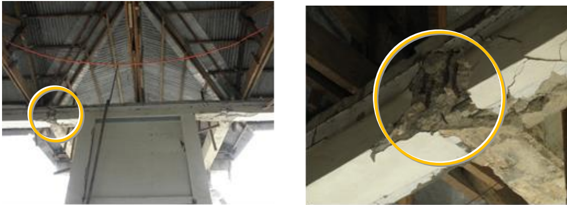
Figure 11. An example of improper structural design in Municipal building of Sagbayan, Bohol (by the earthquake) (Exterior view: refer to Figure 2) (Left) damaged connection of beams of canopy and main structure (Right) Detail of the damage
