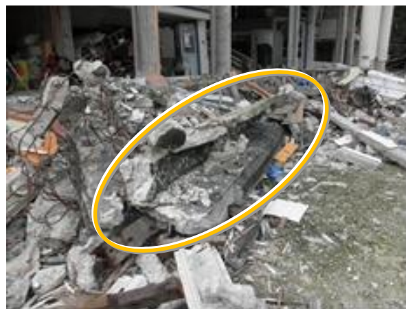
Figure 22 An example of improper installation of concrete gutters in Sagbayan Municipal Office (by the earthquake)
