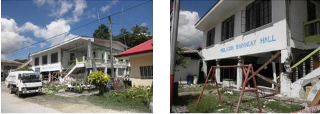
Figure 13 An example of improper structural design in Barangay office in Antequera (by the earthquake): (Left) exterior view, (Right) damaged columns by irregular configuration
