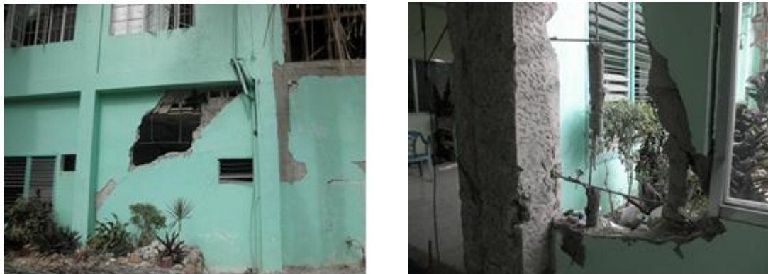
Figure 16 An example of poor quality of concrete hollow blocks (CHB) (by the earthquake): (Left) Damaged non-structural walls in Municipal Office of Catigbian, (Right) Details of a damaged wall.
