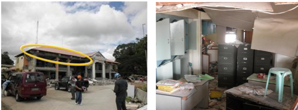
Figure 2. Municipal building of Sagbayan, Bohol: (Left) Heavy damage to shelter walls and so on, and (Right) Inside the buildings
