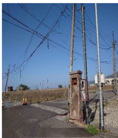
Fig 2: Burnt Power supply line at Wajima
