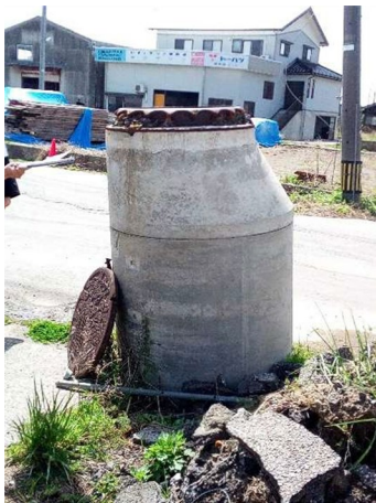
Fig 1: Uplifted Manhole at Suzu
