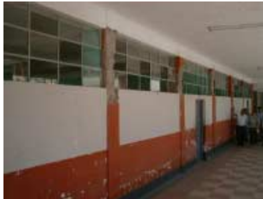
Picture 2-2-3-2. Damaged short column.
