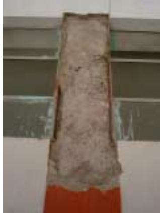
Picture 2-2-3-3. Short column. Wide space between lateral reinforcing bars.
