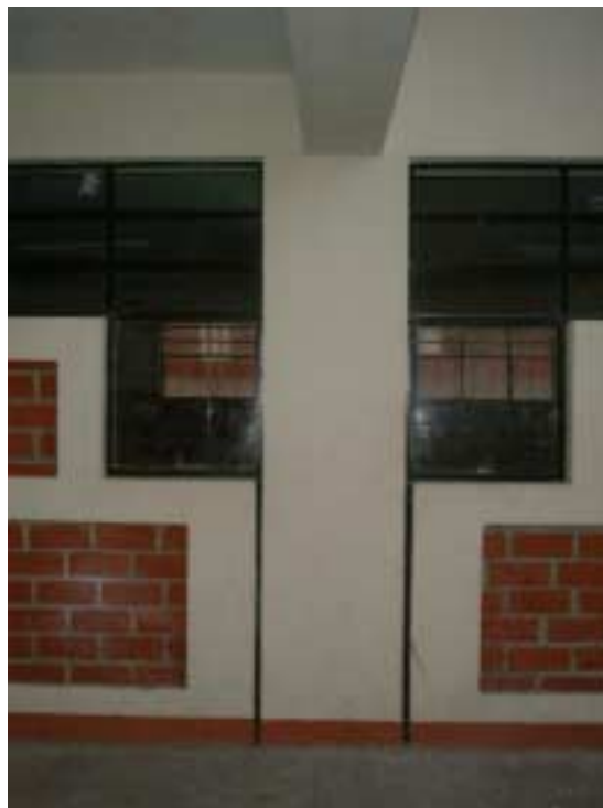
Picture 2-1-5-4. Slit (black part) between the wall and the structural column.
