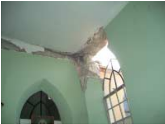
Picture 2-1-4-3. Damaged upper opening. Damaged part where buildings are adjacent and at right angles to each other.
