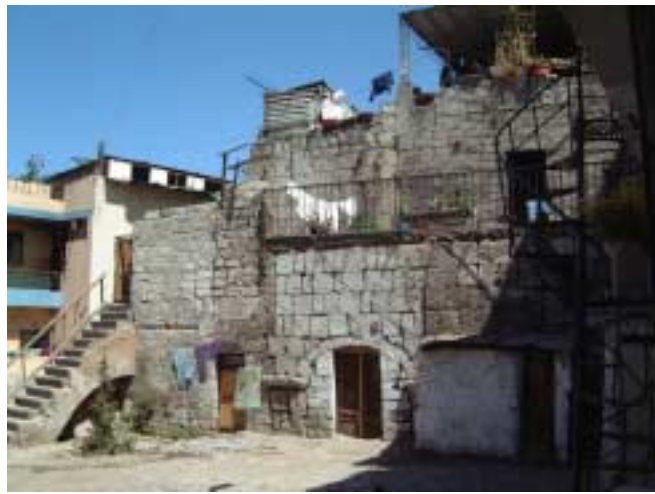
Picture 2-1-8-2. Appearance of the first and second floors. Masonry and brick. Limited damage due to the earthquake but the building is structurally impaired.
