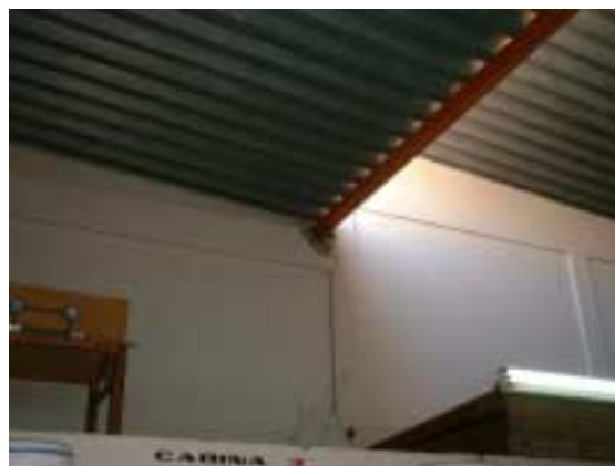
Picture 2-3-2-1. Damaged connection of steel frame with concrete member.
