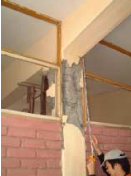
Picture 2.1.2-3. Shear failure of column. Shortened column due to high spandrel wall. Shear reinforcement intervals of 30 cm.
