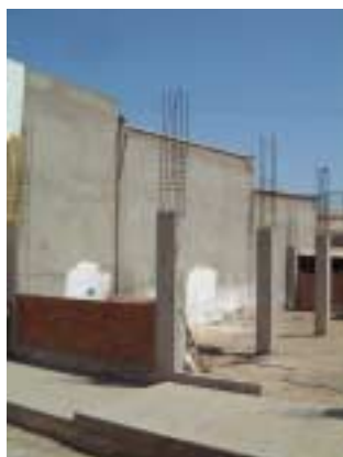
Picture 2-3-2-1. Gable of workshop. Damage at the connection of the steel frame spanning the right non-level part.
