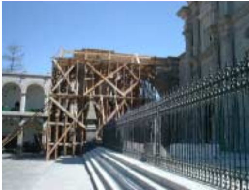
Picture 2-1-7-4. Decorative arches on both sides at the front and loosened due to the earthquake, under repair.
