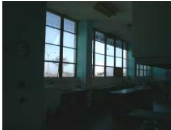
Picture 2-3-6-3. Broken window. Hard putty was used.
