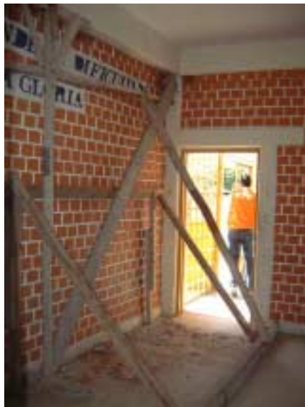
Picture 2-3-7-3. Damaged wall. Emergency support.
