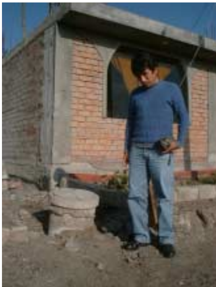
Picture 2-1-3-1. Elevated manhole due to liquefaction.
