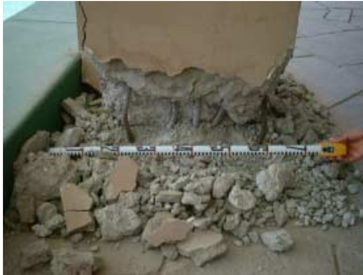
Picture 2-2-9-5. Column base. Buckled main reinforcement.
