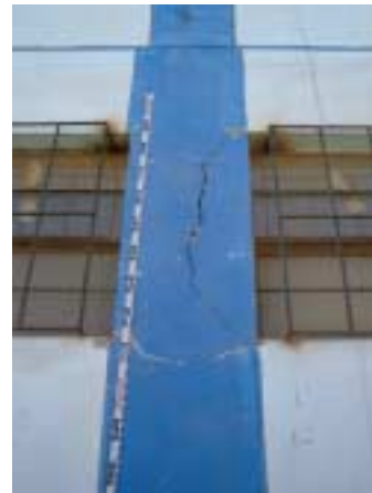
Picture 2-3-4-9. Damaged column. A shear crack was observed in one column.
