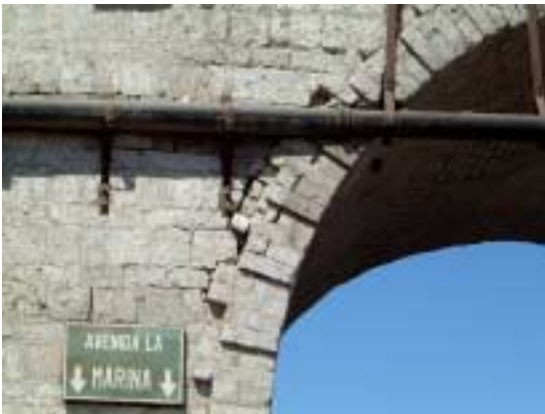
Picture 2-1-6-1. Loosened arch. Loosening between the surface of the arch and other stone masonry was observed.
