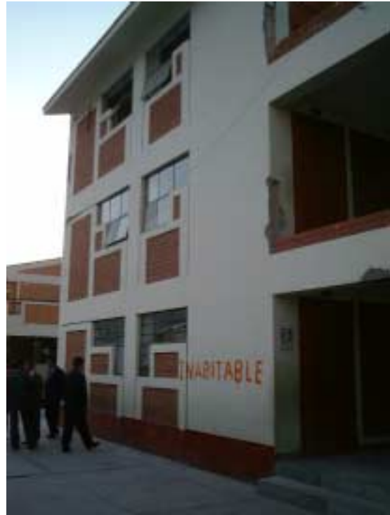
Picture 2-1-5-3. On the near right, the hollow brick walls of the second and third floors can be seen to have collapsed.
