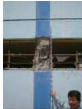
Picture 2-3-4-7. The outside of column on the window side. This column has few lateral reinforcing bars.
