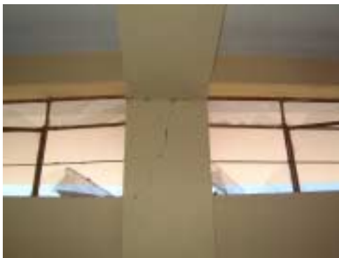
Picture 2-2-4-6. Damaged short column.
