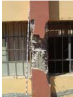
Picture 2-2-4-2. Damaged column.
