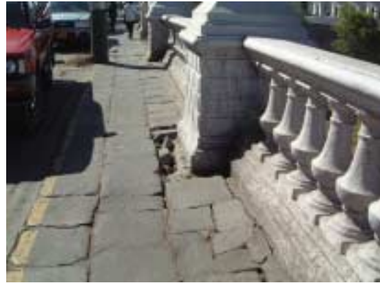
Picture2-1-6-2. Damaged balustrade. Outwardly-displaced balustrade. Road surface showing ripples.
