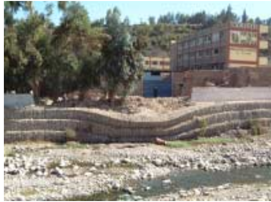
Picture 2-2-2-2. Deformation of the revetments.
