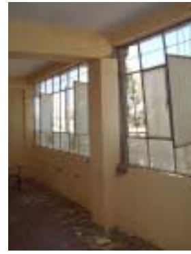
Picture 2-2-4-5. Damaged long column.
