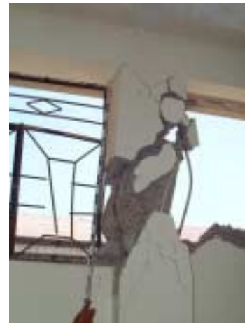
Picture 2-2-3-4. Shear failure of the short column. No lateral reinforcing bar.
