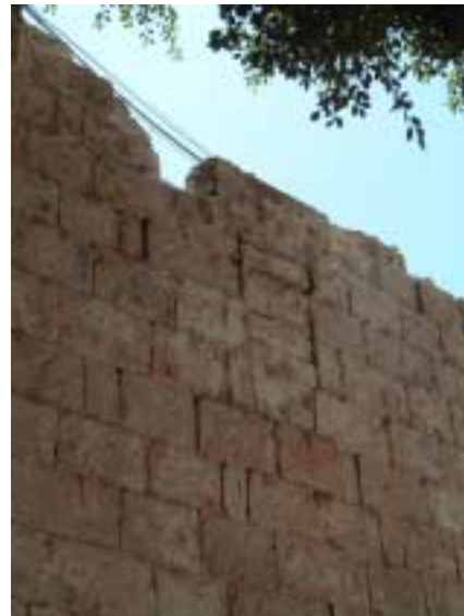
Picture 2-2-6-4. Displaced upper wall.
