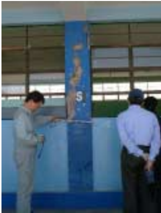
Picture 2-3-4-2. Shear failure of the column on the corridor side resulting from shortened columns due to limited vertical space, occupied by the spandrel wall.
