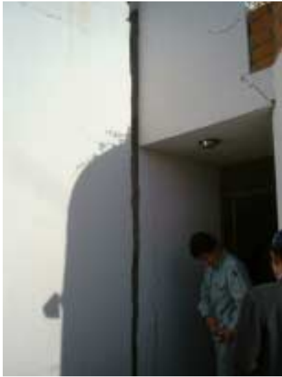
Picture 2-1-3-3. Separated boundary due to the inclination of the building caused by liquefaction.
