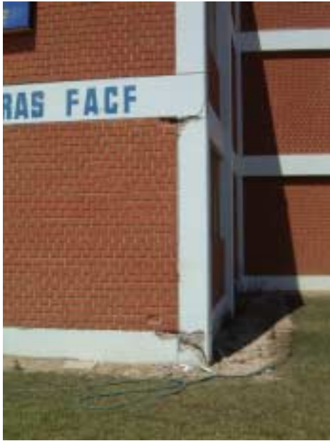
Picture 2-3-7-1. Damaged wall and beam-column joints.
