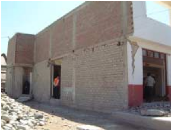
Picture 2-2-3-3. Shear crack in the wall. First floor: concrete block wall. Second floor: brick wall.
