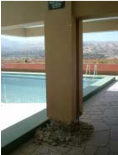
Picture 2-2-9-2. A column supporting a roof slab. Flexural shear failure at column base.
