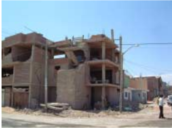
Picture 2-3-5-1. Damaged three-storied building.
