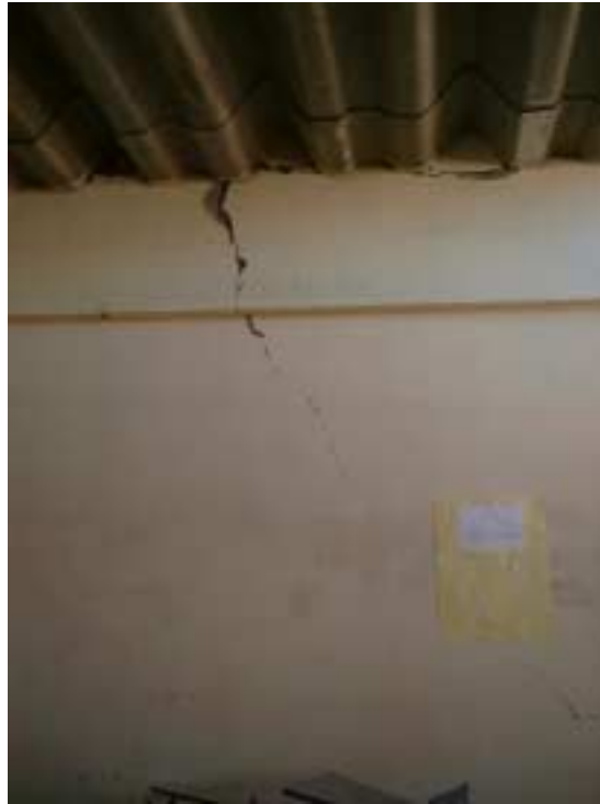
Picture 2-2-3-6. Damaged wall in the span direction.
