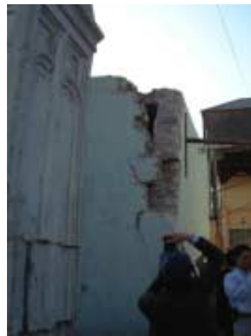
Picture 2-1-4-2. Walls with damaged corners.
