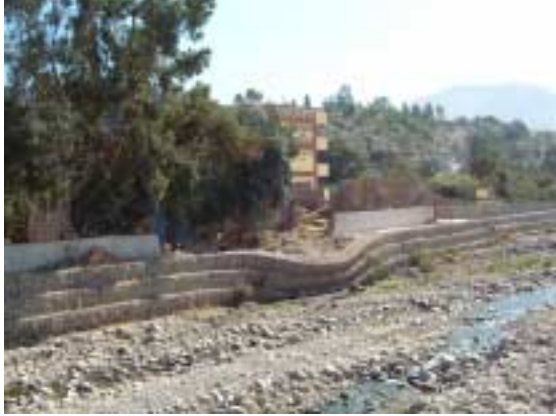
Picture 2-2-2-1. Deformation of the revetments.
