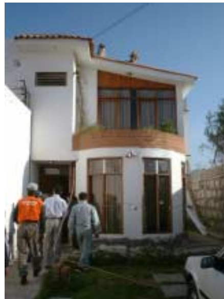
Picture 2-1-3-2. Full view of a building affected by liquefaction.
