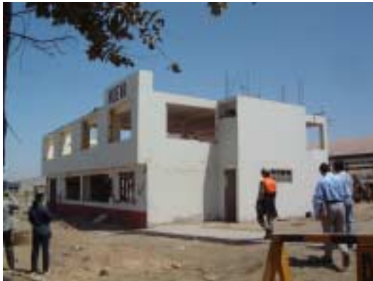
Picture 2-2-3-1. Appearance of the building. The parapet on the rooftop toppled.
