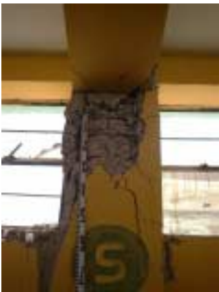
Picture 2-3-4-5. The space between the lateral reinforcing bars of the shortened column measured about 12 cm.
