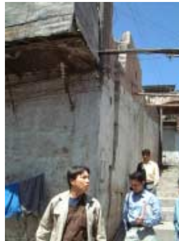
Picture 2-1-8-4. Falling roof arch. Out-of-plane deformation of masonry wall with falling arch.
