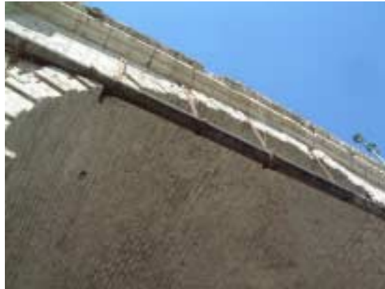
Picture 2-1-6-2. Crack in arch. Crack on the surface of the arch. Some masonry blocks were cracked and displaced.
