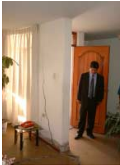
Figure 2-1-3-4. Large cracks in the walls and floors caused by inclination of the building.
