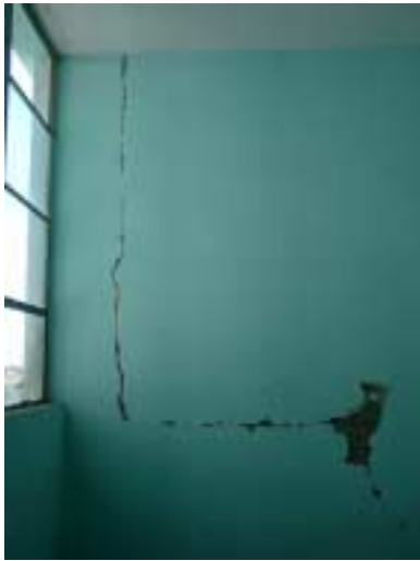
Picture 2-3-6-2. Cracks between nonstructural walls and structural member Crack (stairhall).
