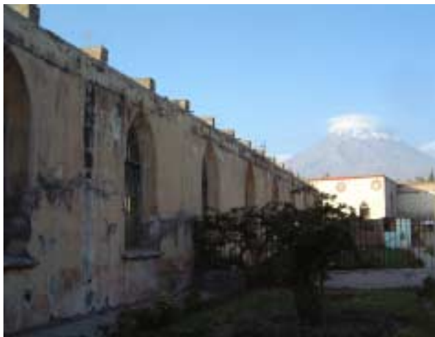
Picture 2-1-4-1. Appearance of the building. Masonry, unique window shape. Beam added to the roof.
