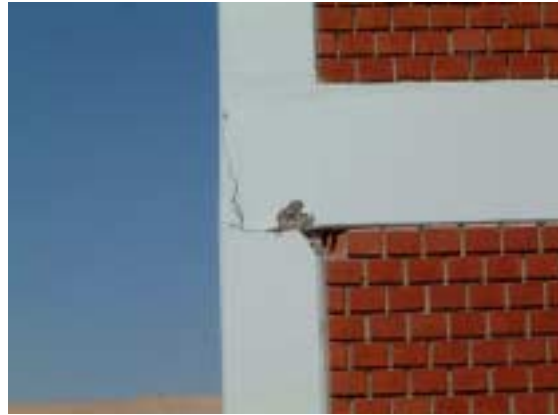
Picture 2-3-7-2. Damaged capital.
