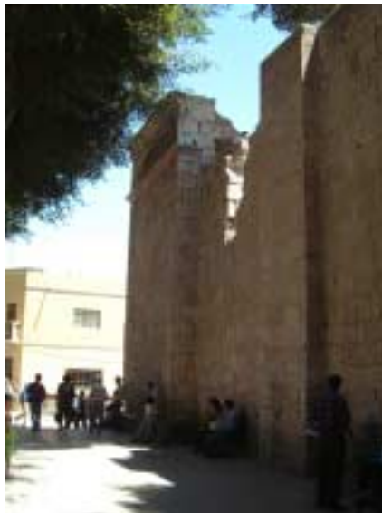
Picture 2-2-6-3. Falling upper wall.
