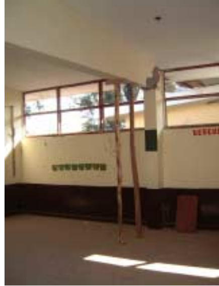
Picture 2.1.2-4. Damaged beam-column joint. Supported with wood.
