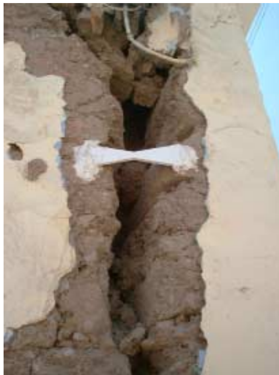
Picture 2-2-5-5. Equipment for measuring increases in crack width, installed by INC.
