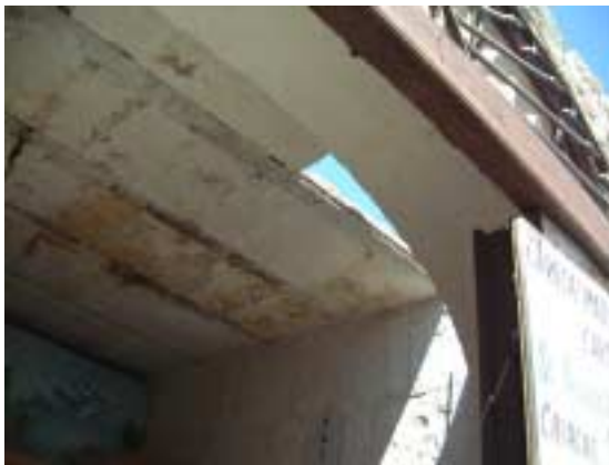
Picture 2-1-8-3. Structure of the top floor roof. Steel rail and sillar roof.
