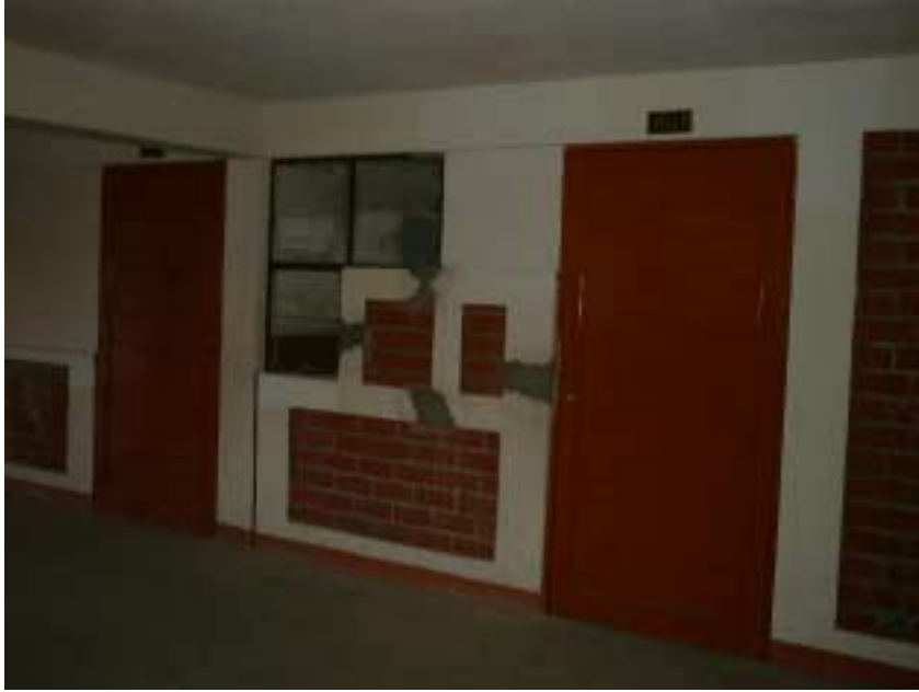
Picture 2-1-5-5. Partial damage to nonstructural walls.
