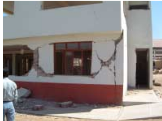
Picture 2-2-3-2. Damaged CB wall and column.
