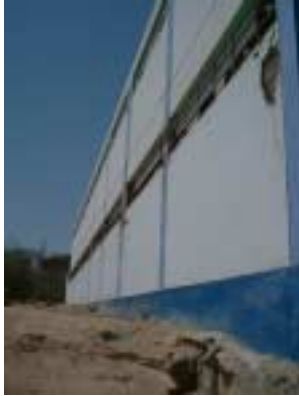
Picture 2-3-4-6. Most columns on the window side of the first floor show shear failure due to their shortness.
