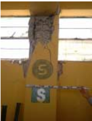
Picture 2-3-4-4. Shear failure of the column on the window side about 35 cm in width.
