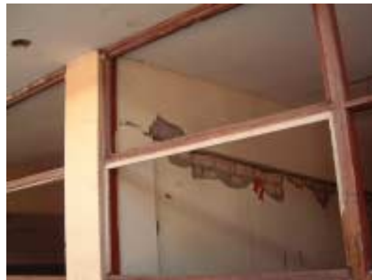
Picture 2.1.2-2. Separation wall in span direction. Damaged capital and beam-column joints. Shear in upper part of brick separation wall.
