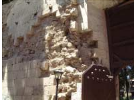
Picture 2-2-6-2. Damage from the earthquake in 1868. The back surface of the wall detached.
