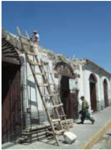
Picture 2-1-8-1. Damage to the top floor. The third floor, facing the road Falling roof eaves.
