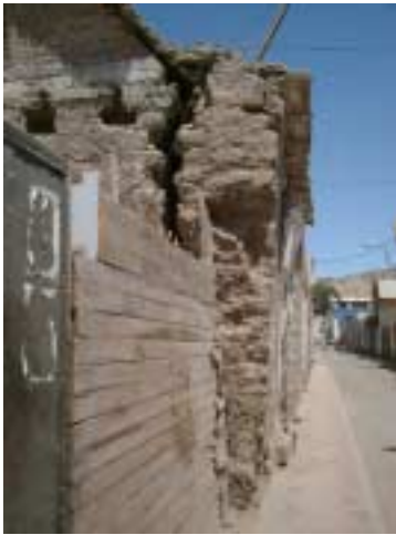
Picture 2-2-5-3. A wall likely to fall out-of-plane. The space widened to this extent in the week after the earthquake.
