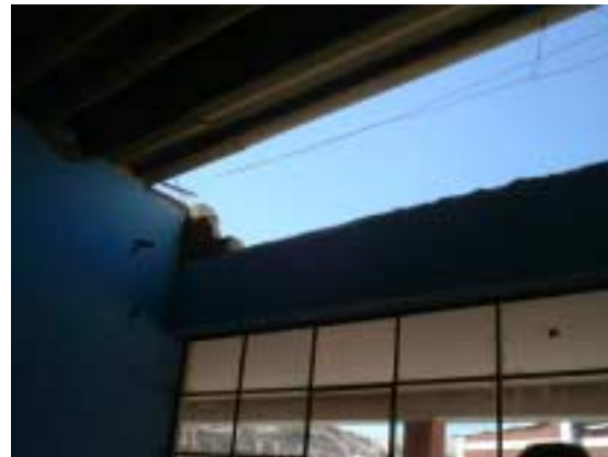
Picture 2-2-3-5. Some of the roof supports collapsed.
