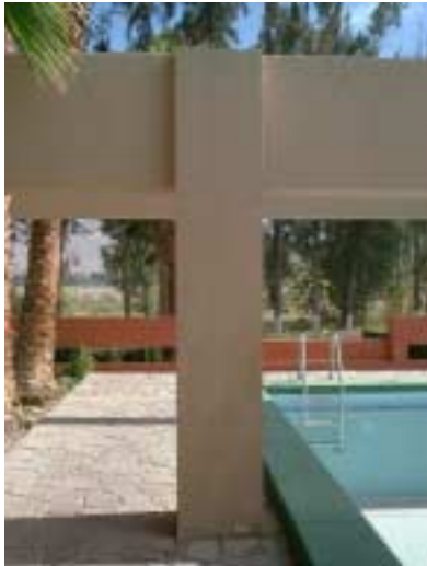
Picture 2-2-9-3. The other column is intact. Flexural cracks are observed in the beam.
