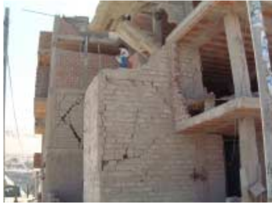
Picture 2-3-5-2. Damaged wall of stairhall The wall of the stairhall on the third floor collapsed.
