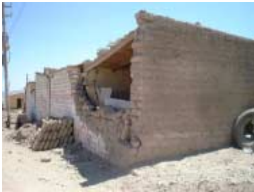
Picture 2-2-7-3. Damaged adobe building. Walls collapsed.
