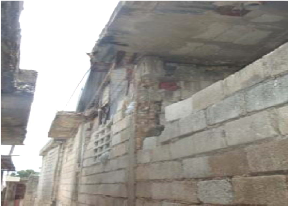
Wall out of plane Failure
