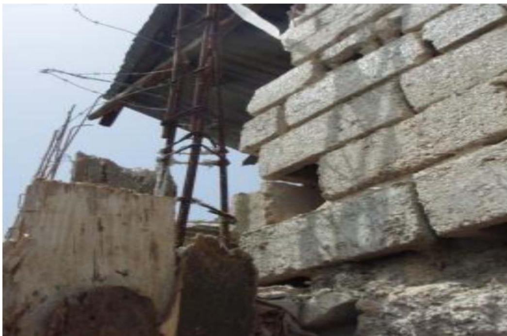
Partially disconnected wall
