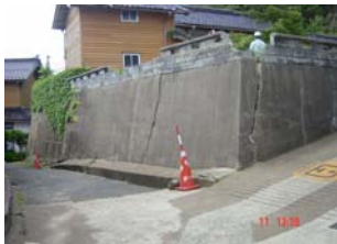
Photo 3 Failure of wall
