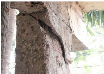
Figure 3. Big shear crack in column.
