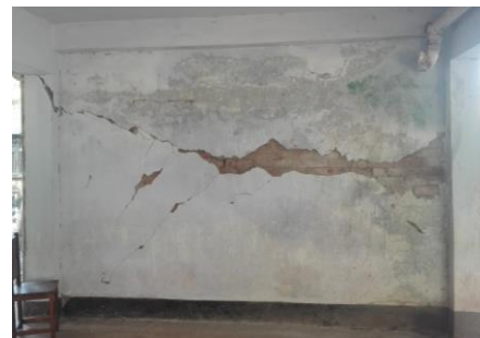
Figure 4. Damaged masonry infill.
