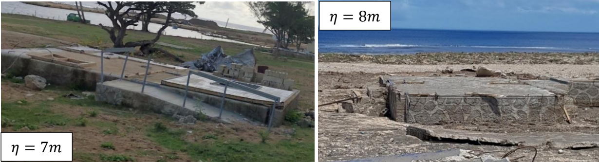
Figure 1: Damaged CRH at ‘Ohonua, ‘Eua with different inundation depth
